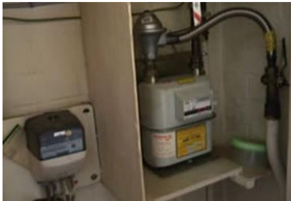
Asbestos panelling around a gas meter
