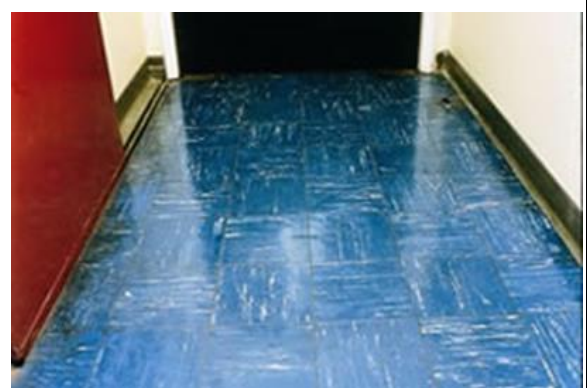
Asbestos containing floor tiles in a corridor
