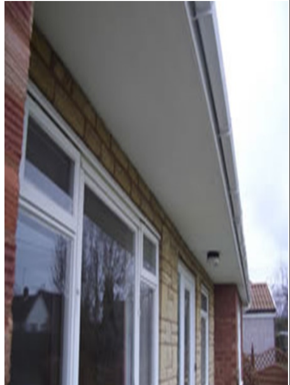
Pieces of Asbestos Insulating Board (AIB)
