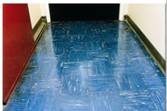
Asbestos containing floor tiles in a corridor
