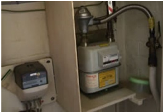
Asbestos panelling around a gas meter
