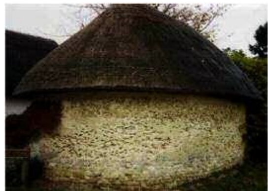
Small thatched witchert stable, the walls are pockmarked by masonry bees, but remain sound and dry under the overhanging thatch and above the unaltered stone plinth
