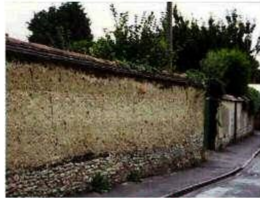
Witchert wall showing three berries above the grumplings. The coping is formed from plain and half round tiles.
