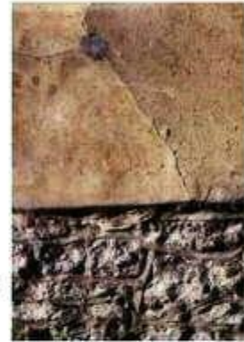
Cement mortar pointed grumplings and cement render. Cracks in both are drawing in water through capillary action. The moisture is unable to escape through dense render and cement mortar.
